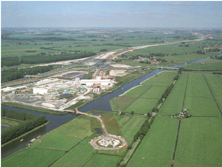
Figure 5 The launching shaft of the Groene Hart tunnel with at the bottom side the first air shaft
